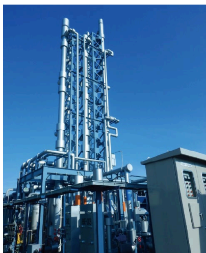
CO 2 Recovery PoC Trial Facility
