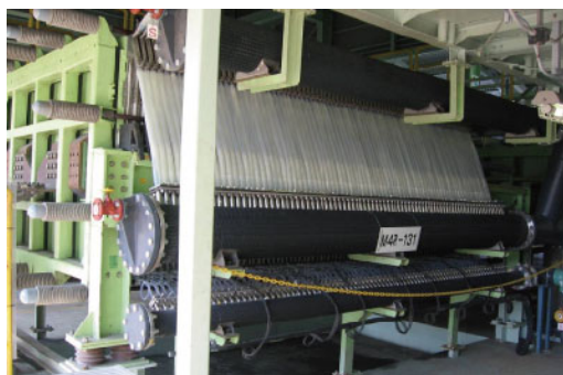
New caustic soda electrolyzer
