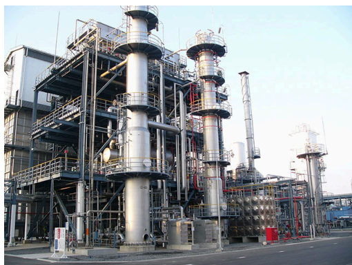
Isocyanate raw material production facility (CO plant)
